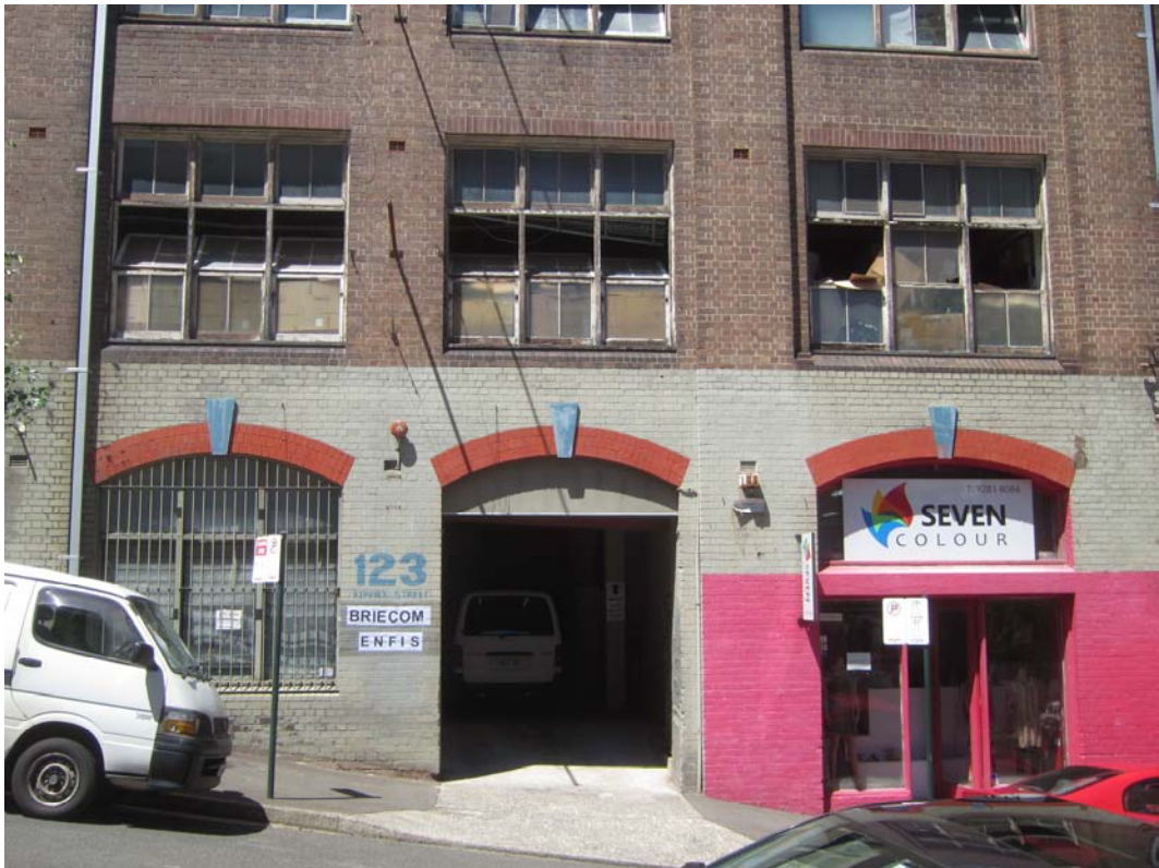
Figure 21 Loading Dock and retail entry on Kippax Street – later modifications to the 1912 building.
